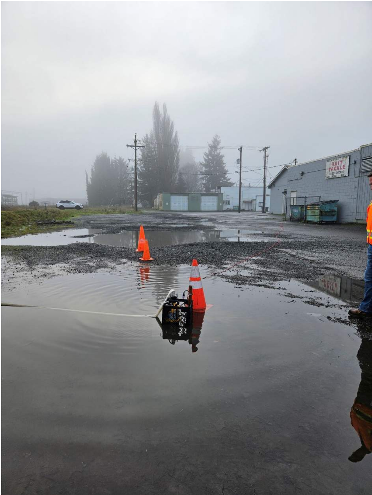
Figure 2. Flooding behind Mini Mart
